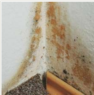
"Since we live in the desert, people have this misconception that if they have a water leak, it will dry up and they won't have a problem.... Mold can take down a home faster than termites."
